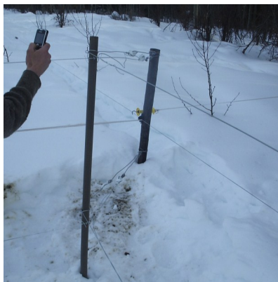
Adding inside fence to exiting fence line at Sandra Burton's in winter 2009
